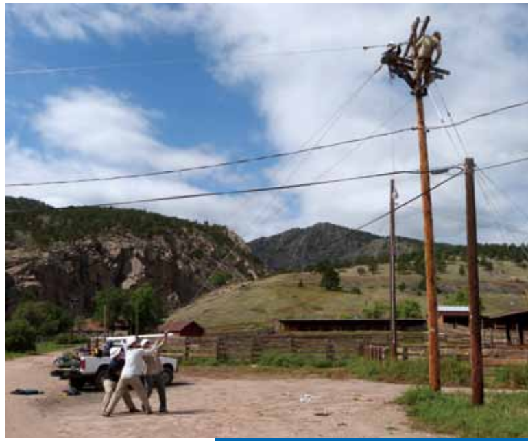
City electric utility employees work to restore power to Sylvan Dale Ranch after flooding in mid-September.
