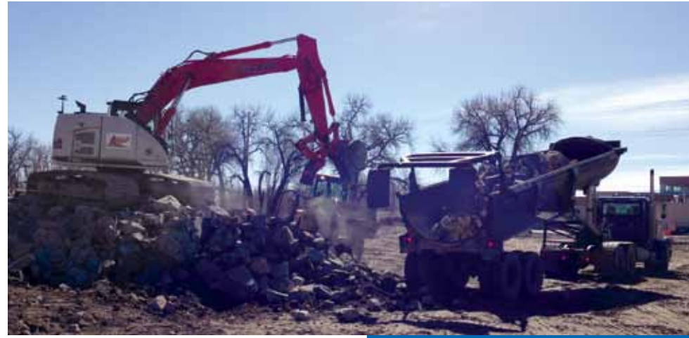
Huge boulders, called rip-rap, are being hauled around Loveland to armor the river banks and, as in this photo from the South Lincoln Avenue bridge project, reconstruct the riverbed.
