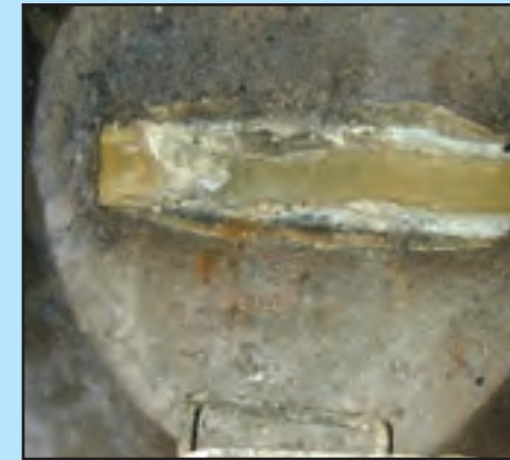
Clogs due to FOG can cause sewer back-ups and create costly repairs for homeowners.
