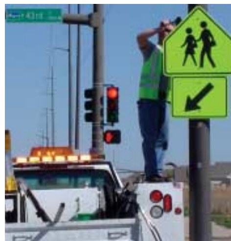
Easier to See - A City staffer installs one of many new school zone signs. Most of the old signs have been replaced this summer. Fluorescent coloring makes the signs more visible to motorists.
